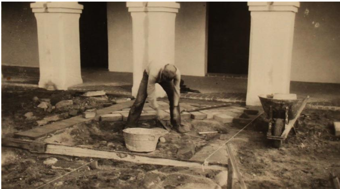
Figure 22: A CCC worker lays bricks for the garden walkways (Frank Pinkley, 1939, Tumacácori National Historical Park Library).
