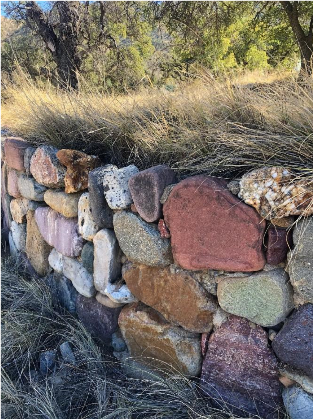
FIGURE 9 - Example of dry stacked stone wall below admin building facing northwest, photo by Melanie Olson, 02/06/21.
